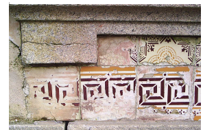
Fig. 3 – PRU 2, showing an extensive loss of glaze.
